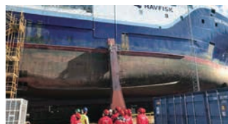
The JSMEA delegation views a trawler having its shelving repaired at VARD Søviknes.
